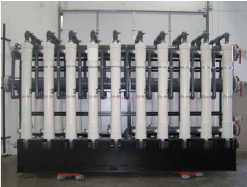
Graywater reuse solutions have used a combination of: filtration, microfiltration, ultrafiltration (shown above), and reverse osmosis.
